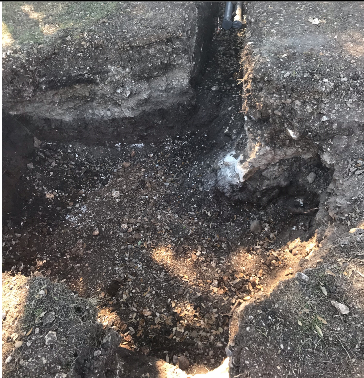
Photograph 4.1: An overview of the excavation in December 2019. Note the fiber optic line at the top of the photo.
